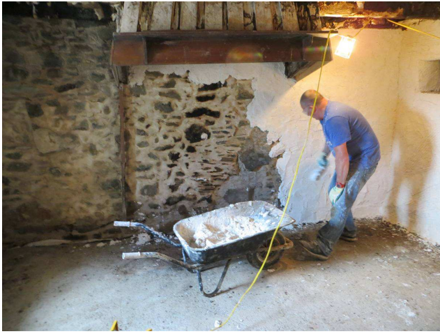
Applying first coat of insulated lime plaster in the kitchen; HES image
