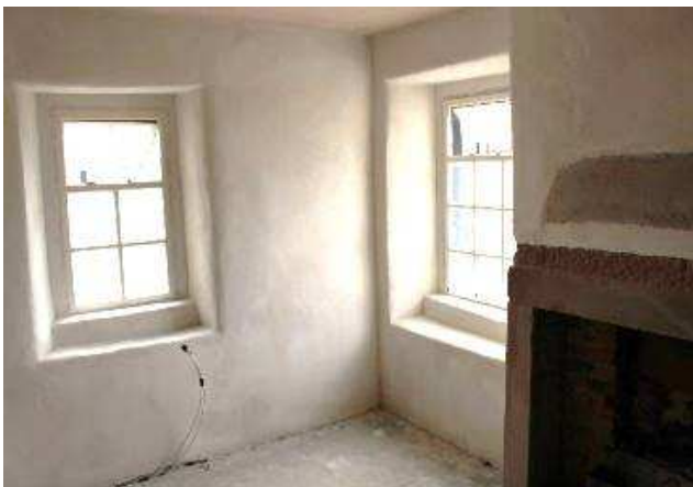
Insulated wall (lime plaster and cork) © Ecological Building Systems
